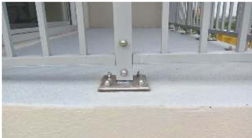
Figure 5 Metallic railing anchored to a concrete slab. Source: (Haukohl et al., 2019)
