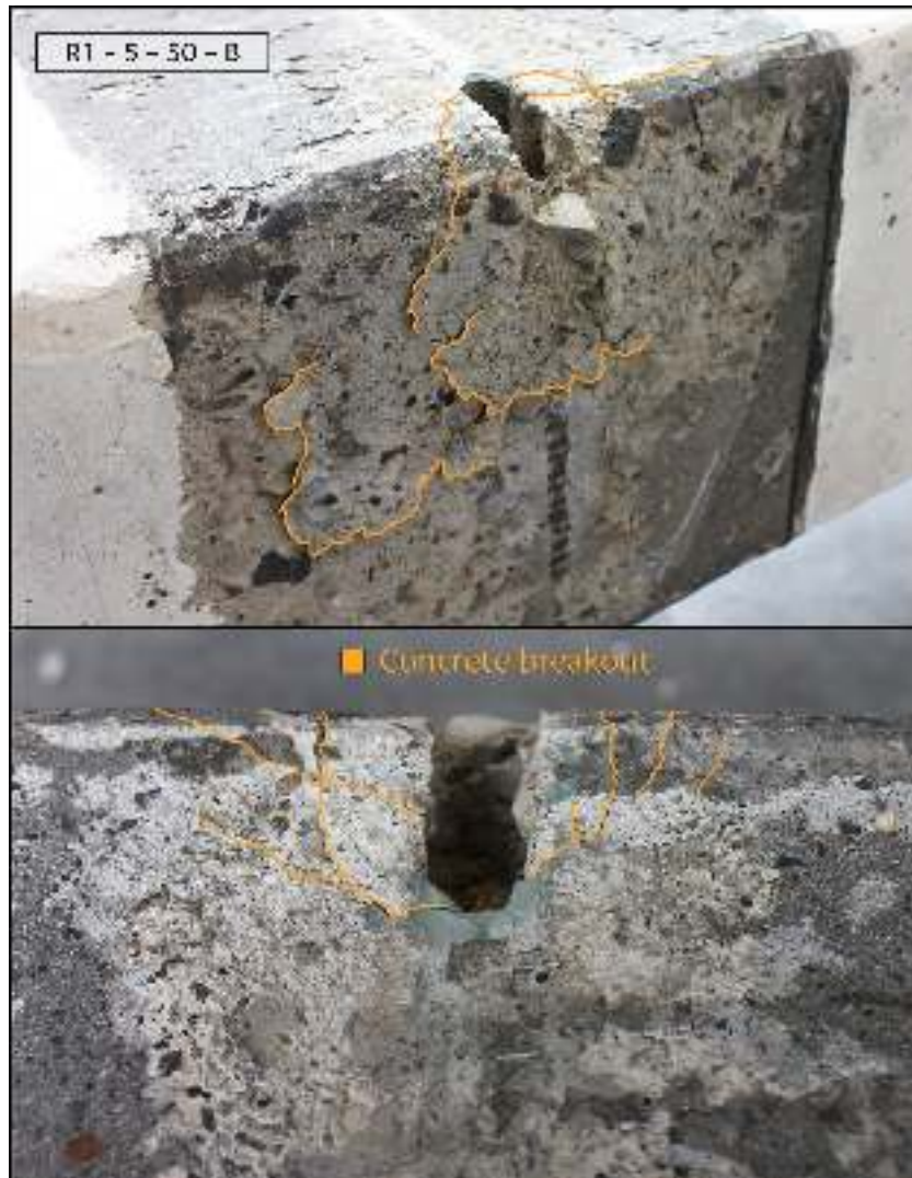
Figure 88 Failure mode R1 – 5 – 50 – B. Source: Own.
