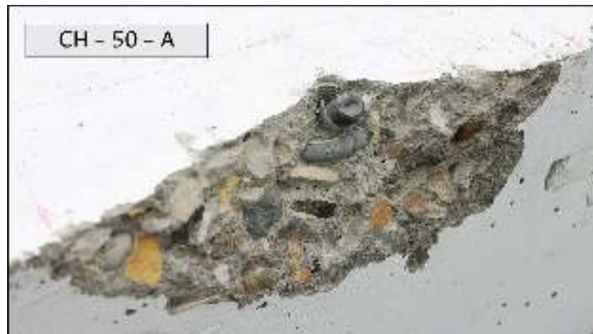
Figure 83 Failure mechanism CH – 50 – A*. Source: Own.
