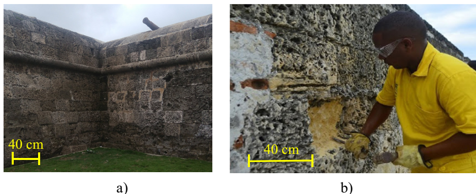
Fig. 1. a) Widespread deterioration in a Structure section; b) Stone replacement process on the Cartagena walls.
