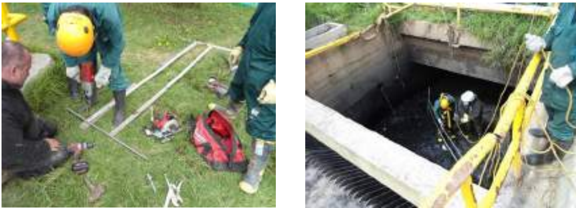
Figure 3.20 Structure 2: sensors installation inside the discharge tunnel.
