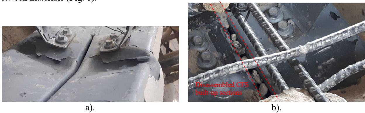
Figure 8. Final state of self-drilling screws fastening system. a). Local buckling on CFS shapes. b). Separation in closed built-up section.
